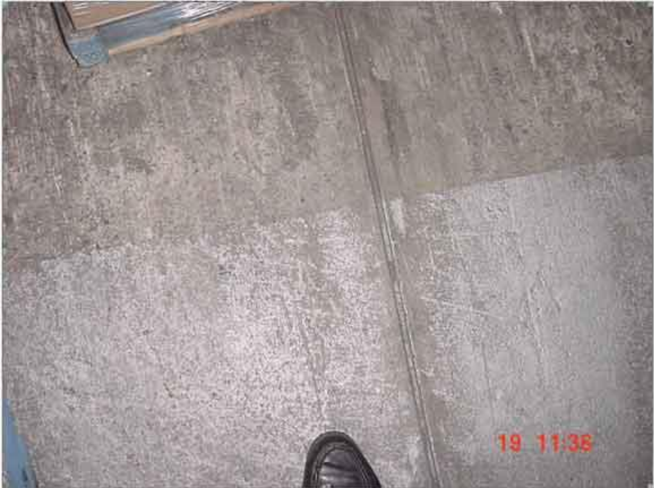
528 Rust Grip bottom; top unsealed concrete
