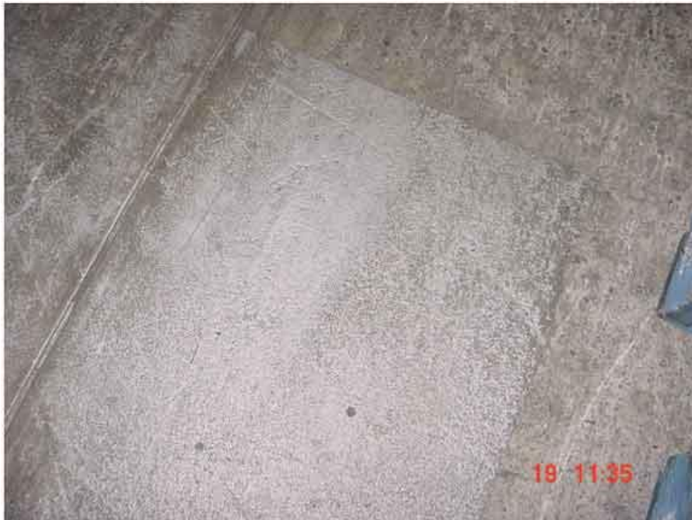
Photo 526 concrete still sealed the color gone
