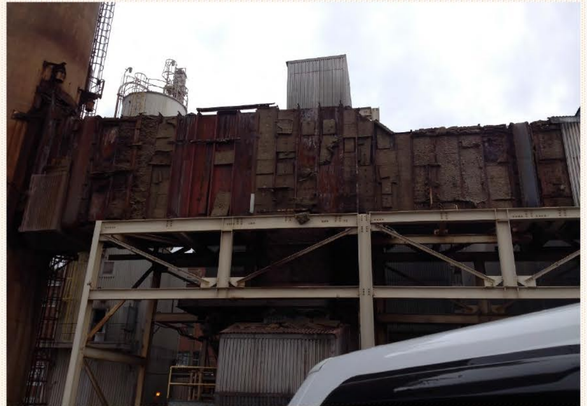
Corrosion Under Insulation and Acid Dew Point Corrosion
