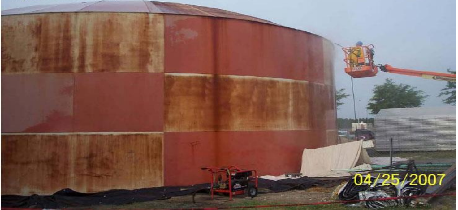
Simmons Army Airfield – 2007 Ft. Bragg, North Carolina Deluge Tank #1 (Dome Roof) Rehab Lead-Base Paint Encapsulation using Rust Grip®
